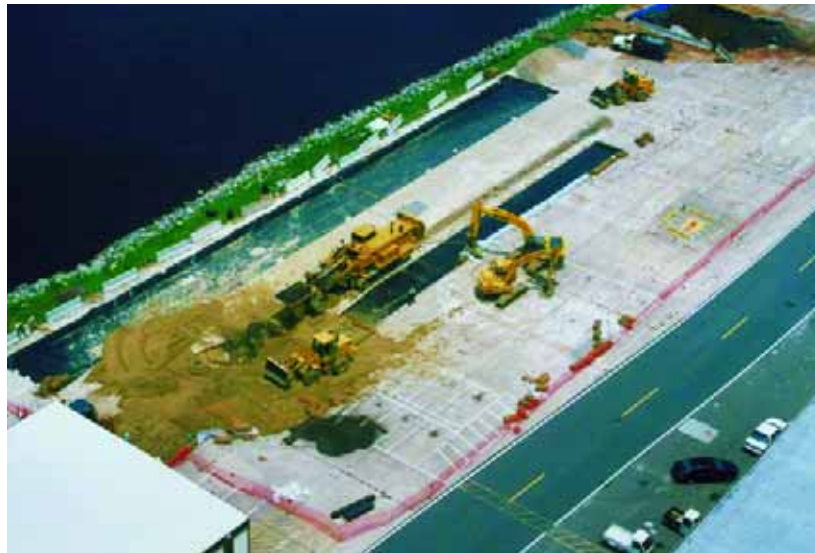
An installation of a permeable reactive barrier for the treatment of contaminated groundwater. Photo courtesy of professor David Blowes
