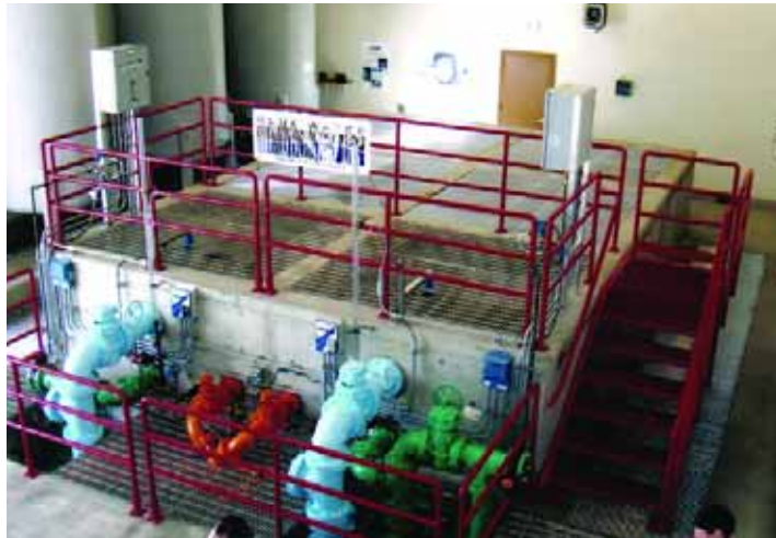
Interior of the new wastewater research facility in Hayden, Idaho. Photo courtesy of Blue Water Technologies Inc.
